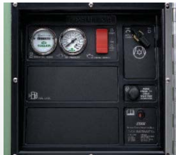
Curbside Instrument Panel with (SSAM) Shutdown System & Annunciation Module.
